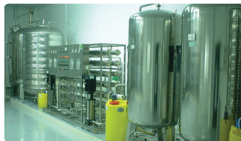
Water purification system
